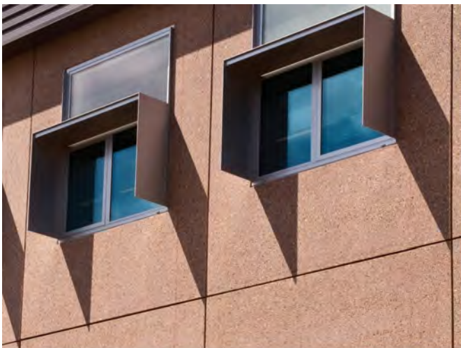
Eastern/Western orientation response: National Renewable Energy Laboratory RNL Golden, Colorado, United States Credit: Dennis Shroeder / NREL
